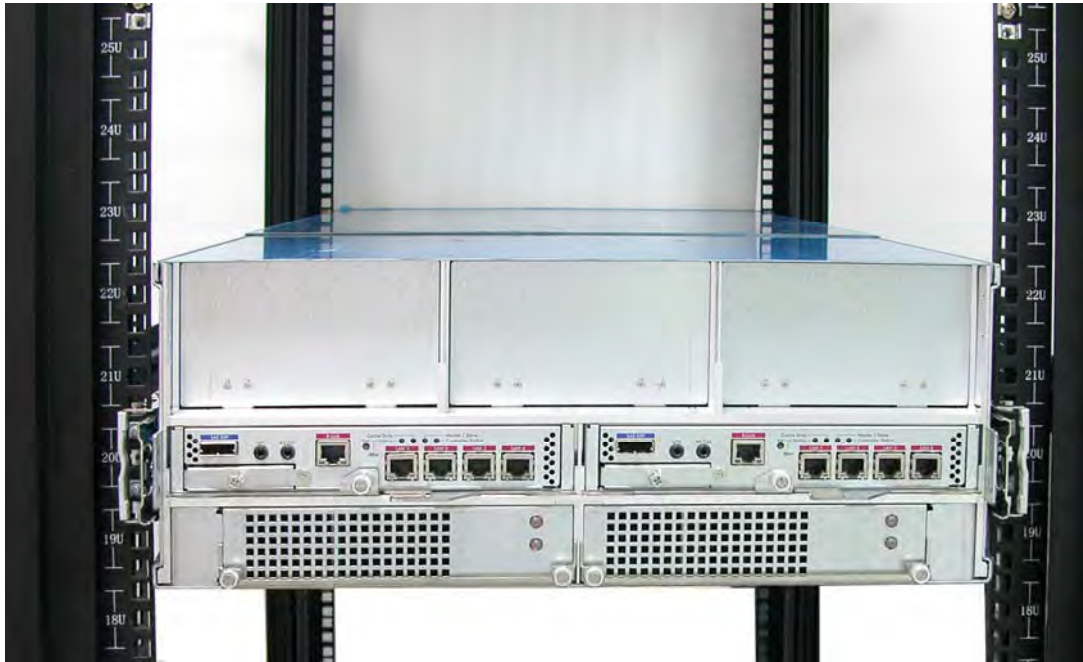
View from Rear Side of Rack Cabinet Enclosure is Pushed Inwards
